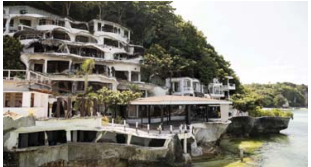
A general view shows the almost demolished West Cove Hotel on the Philippine island of Boracay.
