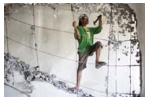
A worker demolishes a wall of the West Cove Hotel on the Philippine island of Boracay.
