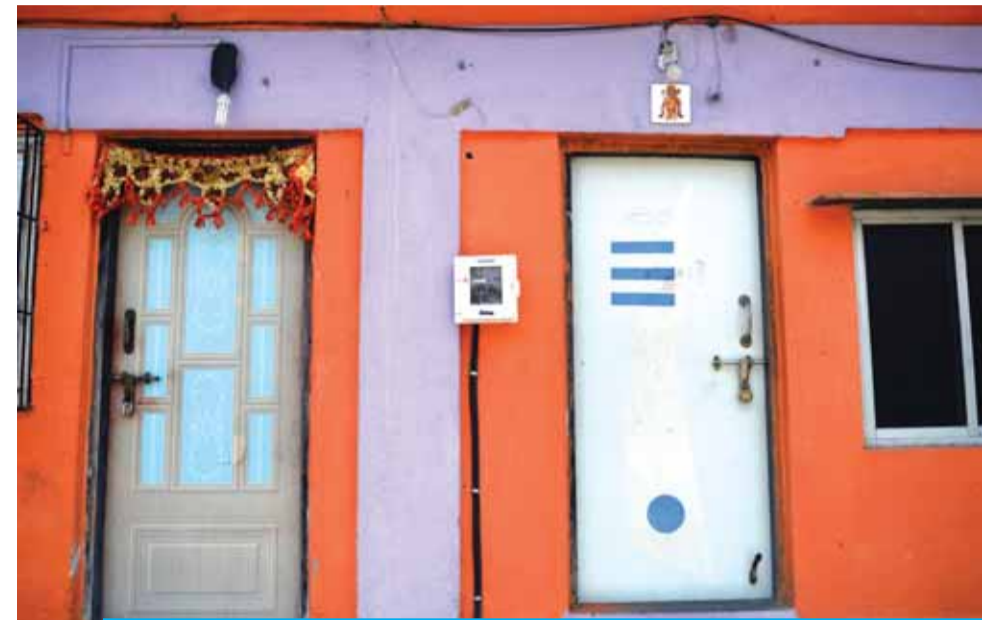
MUMBAI: This photo taken on March 9, 2018 shows an electricity supply metering board on a wall of houses in a village on Elephanta Island near Mumbai. —AFP
