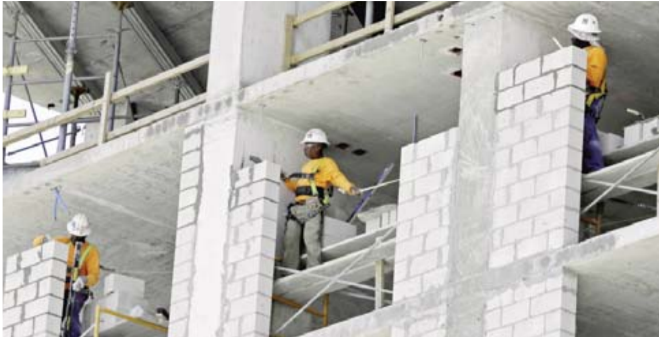
MIAMI: In this May 4, 2017 photo, construction workers work on an apartment high rise in Miami. The Commerce Department issued the third and final estimate of how the US economy performed in the April-June quarter. — AP
