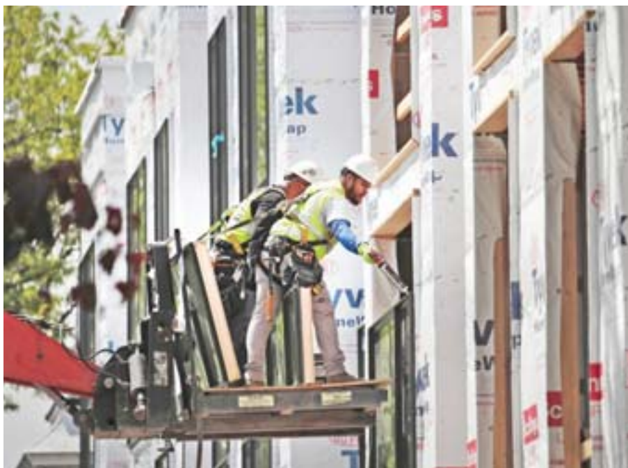
CHICAGO: This file photo taken on May 14, 2017 shows workers installing windows in a townhome complex under construction in Chicago, Illinois. — AFP
