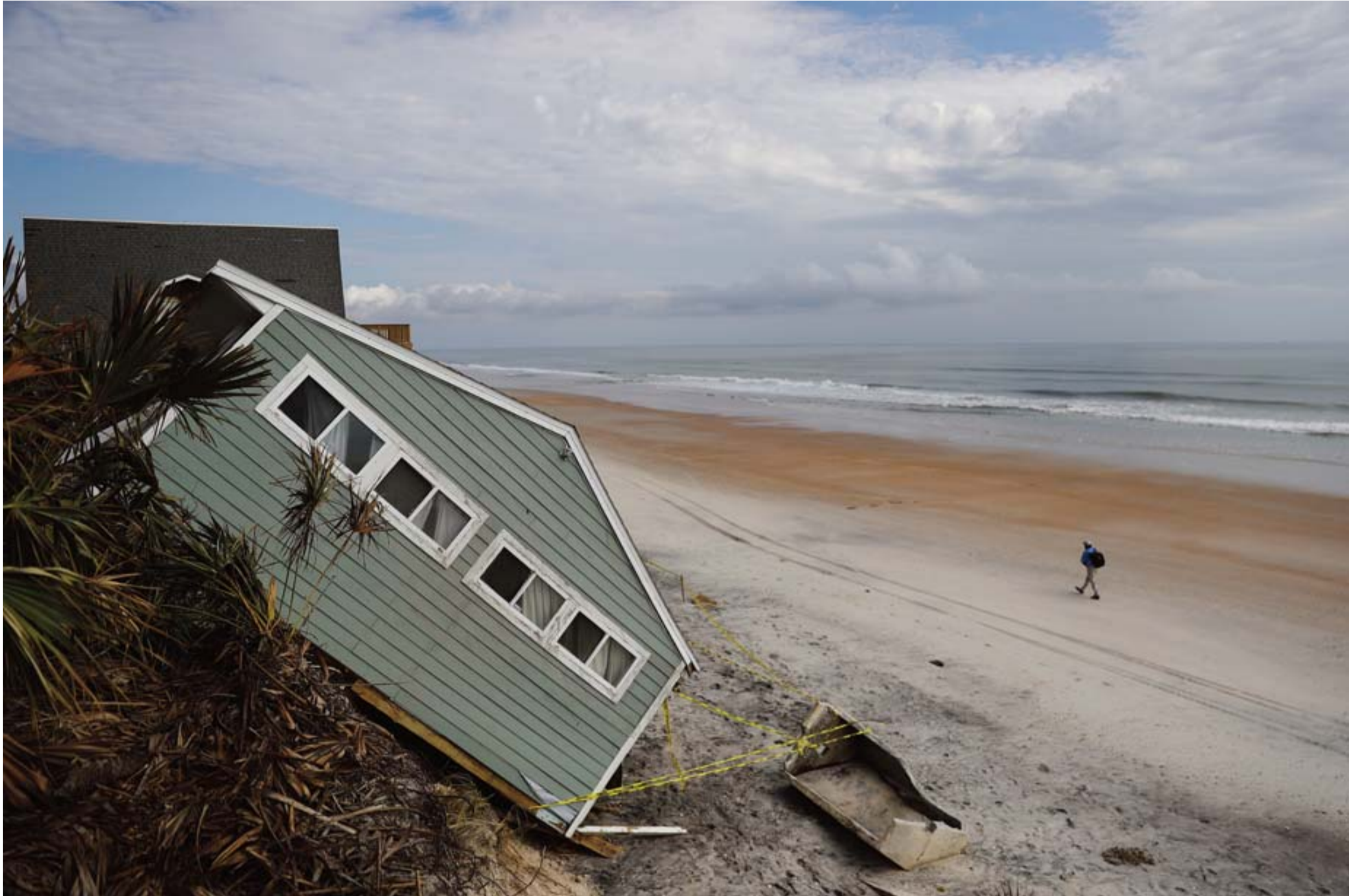
VILANO BEACH: A house rests on the beach after collapsing off a cliff from Hurricane Irma in Vilano Beach. — AP
