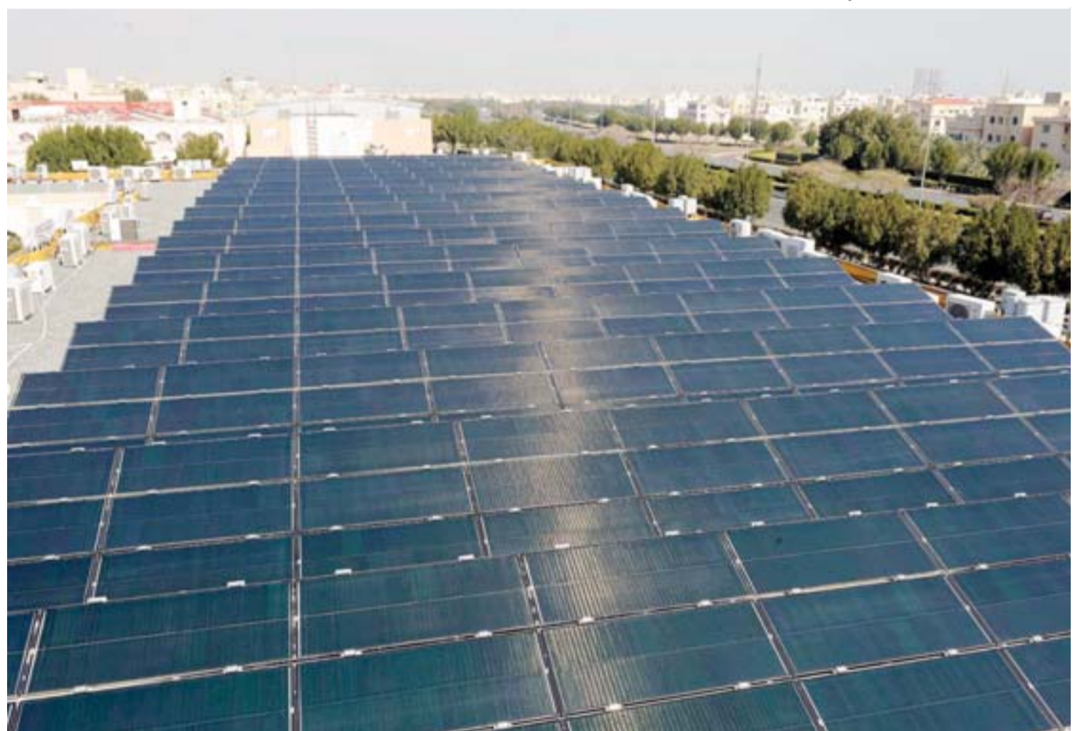
Solar panels to produce energy for schools.
