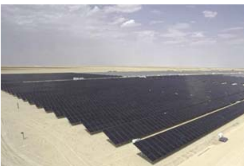
Solar panels at Al-Shaqaya Renewable Energy Complex.
