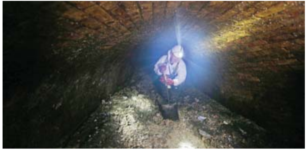
LONDON: This file photo shows a Thames Water sewer supervisor working in the intersection of the Regent Street and Victoria sewer in London. — AFP
