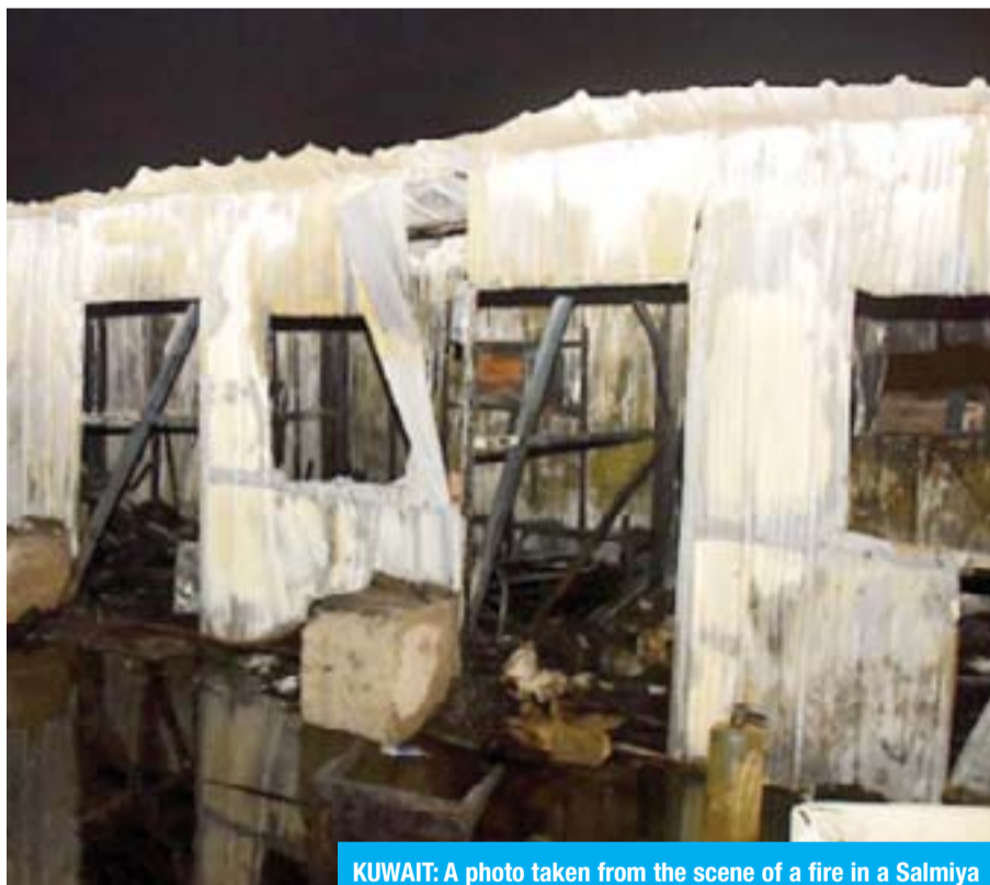
KUWAIT: A photo taken from the scene of a fire in a Salmiya hotel after it was extinguished.
