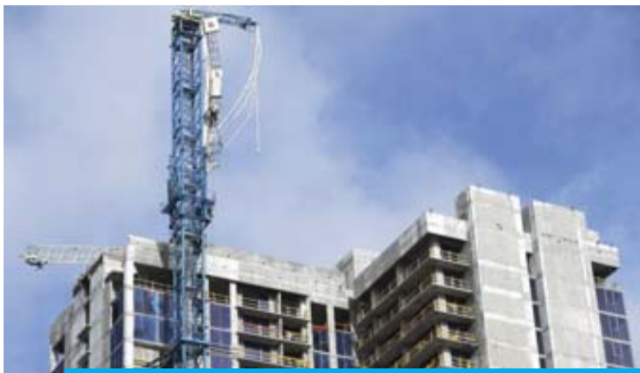
MIAMI: This file photo taken on September 11, 2017 shows a broken crane caused by winds from Hurricane Irma sitting on top of a building under construction in downtown Miami, Florida. — AFP
