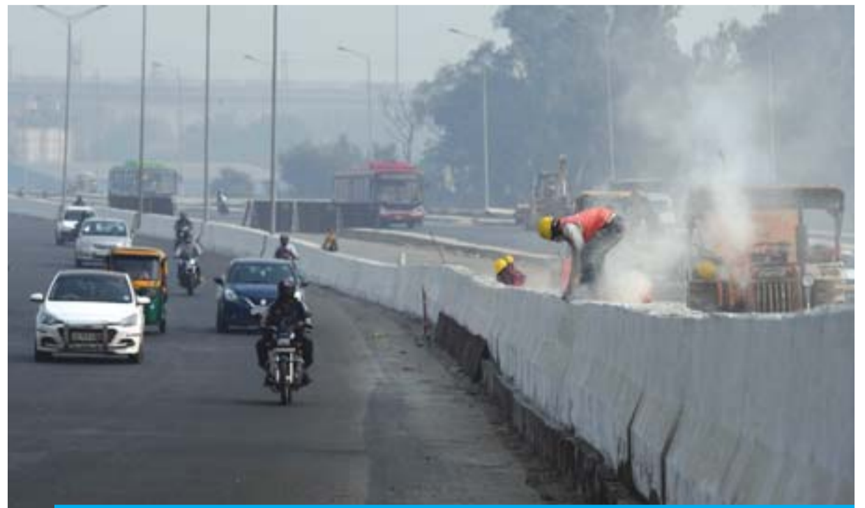
NEW DELHI: Dust billows as a worker grinds the concrete divider of an under-construction flyover as vehicles drive through a smog covered New Delhi yesterday. Delhi is now the world's most polluted capital according to the WHO, with pollution levels that regularly exceed those of Beijing. —AFP
