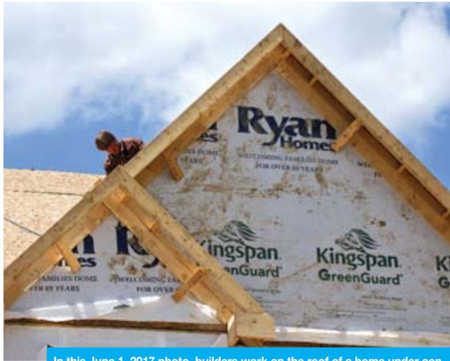
In this June 1, 2017 photo, builders work on the roof of a home under construction at a housing plan in Jackson Township, Butler County, Pa. — AP
