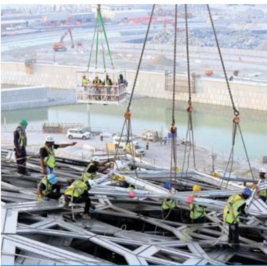
Workers placing the final piece of the outer cladding of the dome structure of the future Louvre museum on Saadiyat Island.
