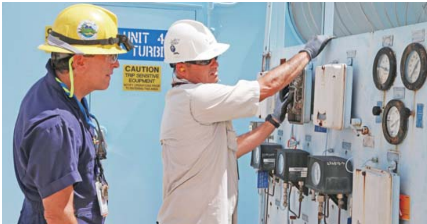
HOMESTEAD: Juan Madruga, left, and Pehter Rodriguez, right, of Florida Power and Light work on the Turkey Point Nuclear Reactor in Homestead, Florida.
