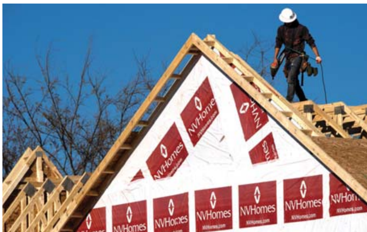
FAIRFAX: This file photo taken on March 8, 2017 shows a construction worker installing a rooftop on a new home being built in Fairfax, Virginia. — AFP
