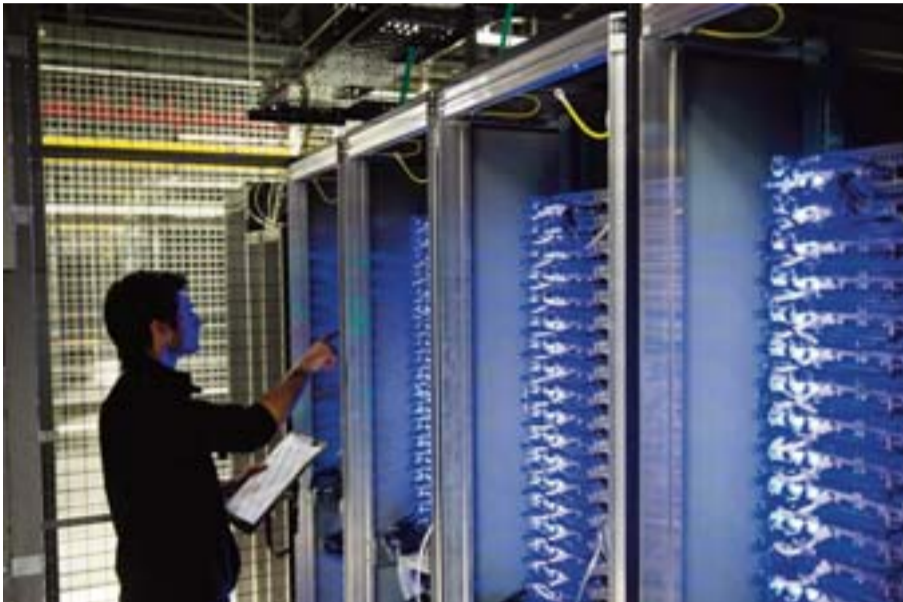
This photo taken on July 21, 2014 shows an employee of Equinix data center checking servers on July 21, 2014 in Pantin, a suburb north of Paris in the Seine-Saint-Denis department. —AFP
