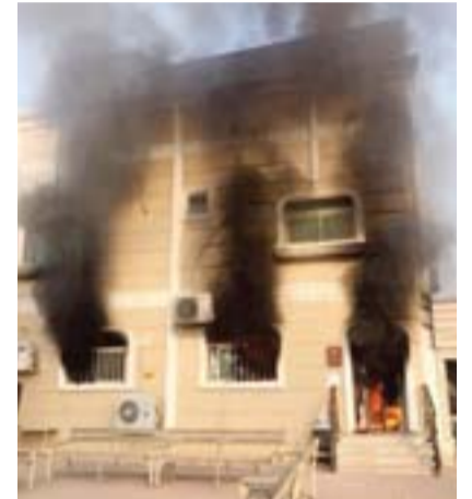
Smoke coming out from a burning house in Oyoun.
