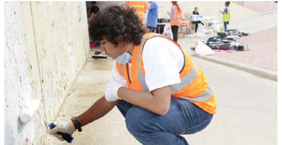
A kid volunteers in an activity to paint the walls of Jabriya-Rumaihiya tunnel.
