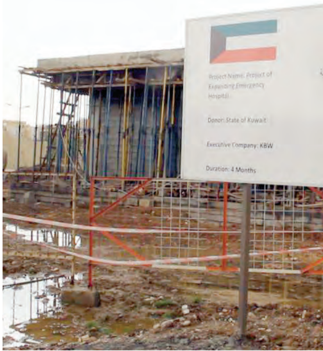
IRBIL: A picture taken during the construction of the 'Kuwait Ward' at Irbil's Emergency Hospital. — KUNA
