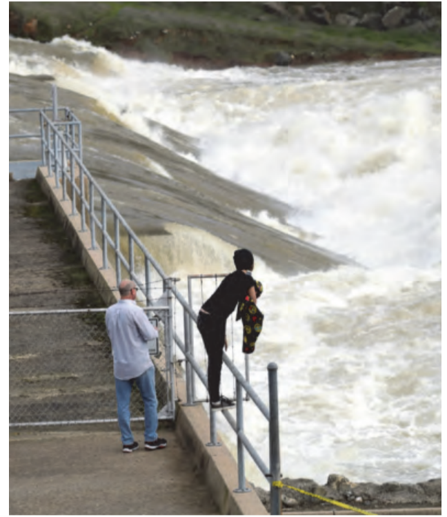
OROVILLE: In this Feb 15, 2017, file photo, people watch the gushing waters of the Feather River from the town's fish hatchery a day after an evacuation was lifted in Oroville, California. — AP
