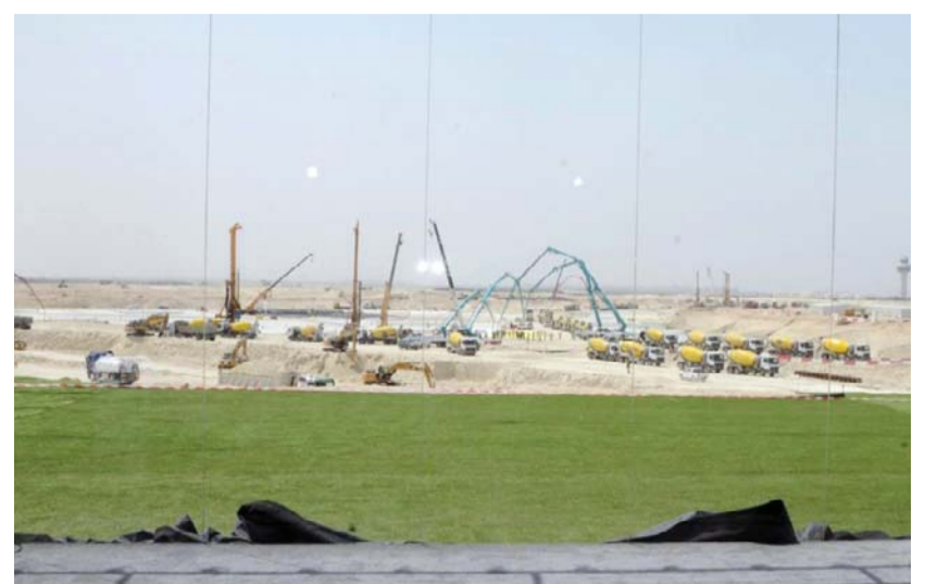
Ongoing construction works at the site of the new Kuwait International Airport terminal.
