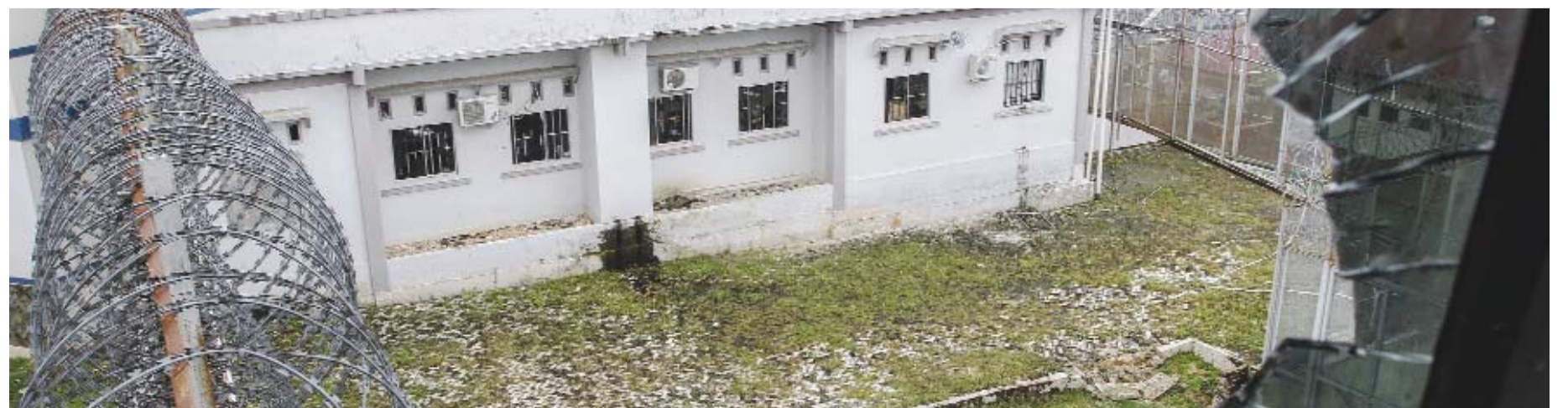
RIAU PROVINCE: Prison buildings are seen through a broken window at Sialang Bungkok Prison in Pekanbaru, Riau province, Indonesia yesterday. — AP
