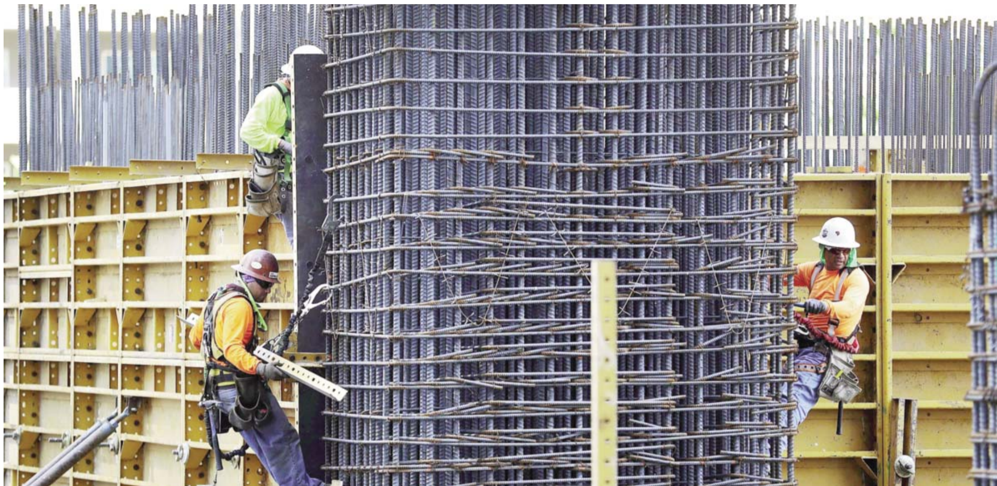
MIAMI: Construction laborers work at a site in Miami, Florida. New claims for US jobless benefits rose more than expected last week, to the highest level in two months, but continued a record low run. — AFP
