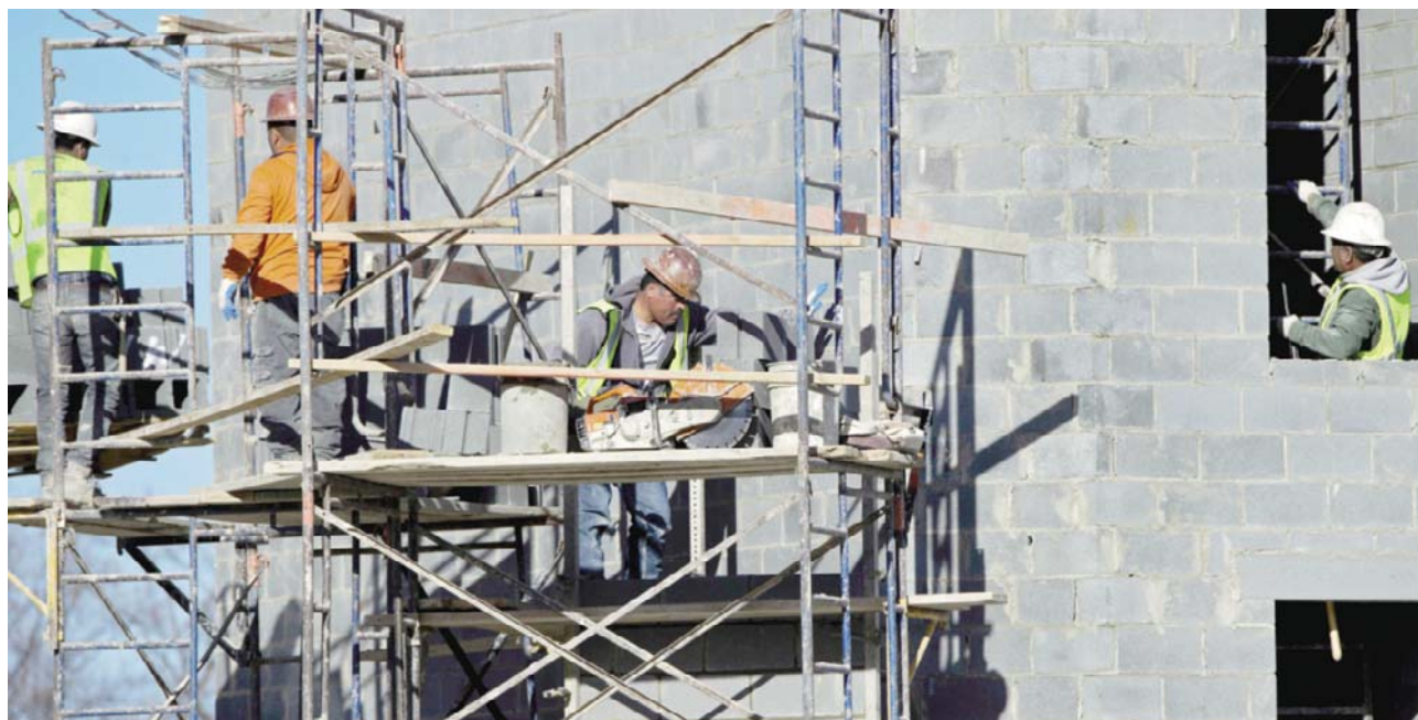
FAIRFAX: Construction workers are seen as they build an apartment building in Fairfax, Virginia. The US housing market, a key economic driver, is exceedingly tight, with supply struggling to meet demand as the sector recovers a decade after the housing crisis, analysts say. —AFP
