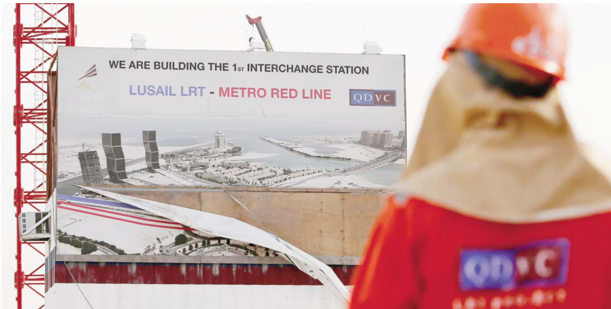
DOHA: This file photo taken on March 24, 2015 shows a worker of QDVC (Qatari Diar/VINCI Construction Grands Projets), the Qatari branch of French construction giant Vinci, walking at the construction site of a new metro line in the capital Doha. — AFP Photos
