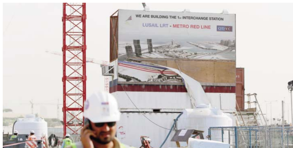
DOHA: Qatar's metro, once completed, will run hundreds of kilometres across ultra-modern Doha, along the coast and into its expanding suburbs. But whether car-mad Qataris will actually use it remains an open question.
