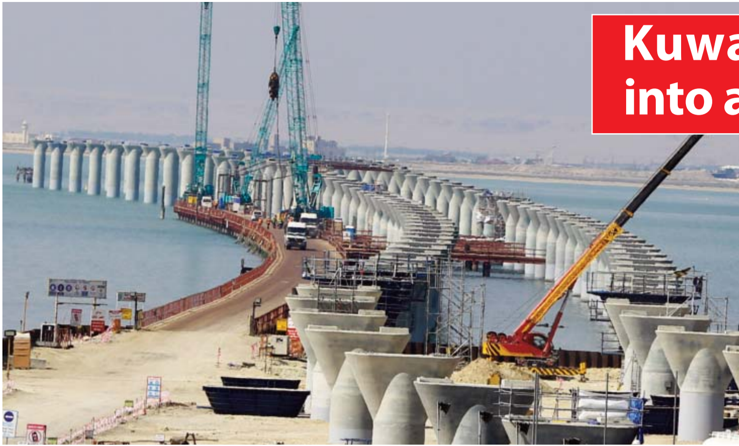
This file photo taken on February 11, 2017 shows a general view in Kuwait City of a construction site of the Sheikh Jaber Al-Ahmad Al-Sabah causeway.
