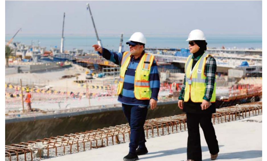
KUWAIT CITY: Ahmad Al-Hassan (left), assistant undersecretary for road engineering at the public works ministry and project engineer Mai Al-Messad walk at the construction site of the Jaber Causeway in Kuwait City on February 11, 2017. —Photos by Yasser Al-Zayyat
