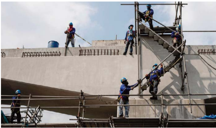
MANILA: Workers are seen on scaffolding at a construction site for an expressway in Manila yesterday. — AFP
