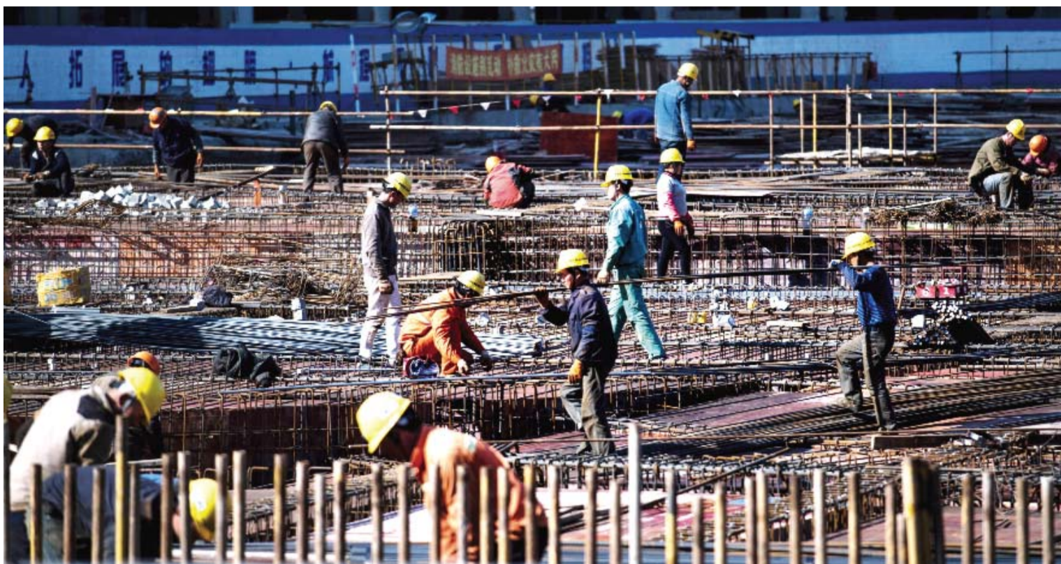
SHANGHAI: Workers are seen on a construction site of a high rise building in Shanghai yesterday. —AFP
