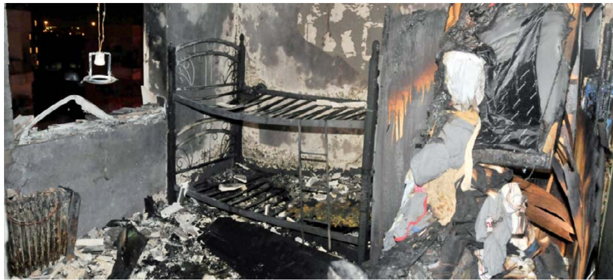
KUWAIT: Damage left by a fire reported in a Khaitan apartment Saturday night.
