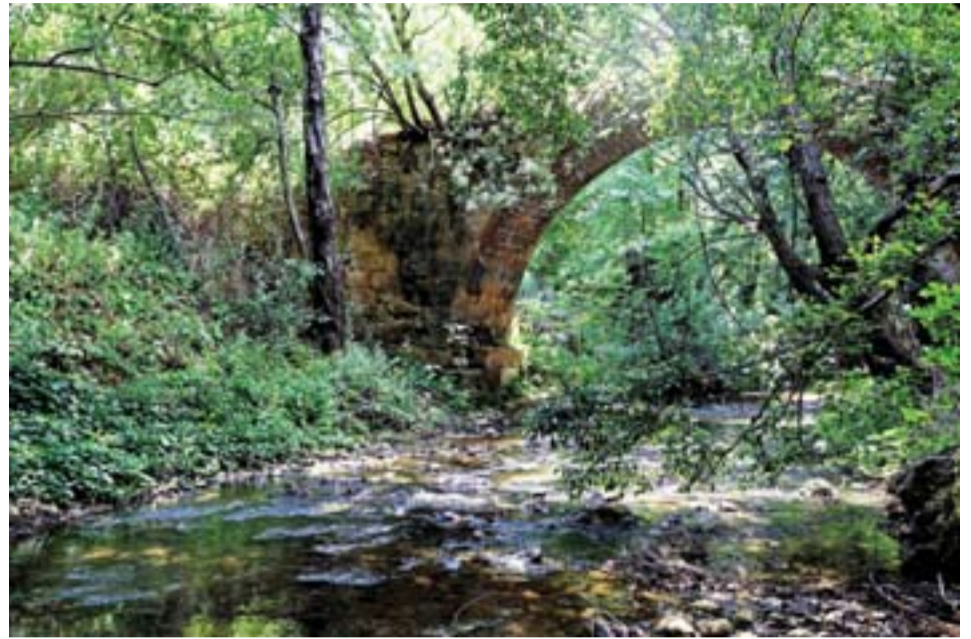
A Roman built bridge which was renovated during the Ottoman rule over the Bisri river .
