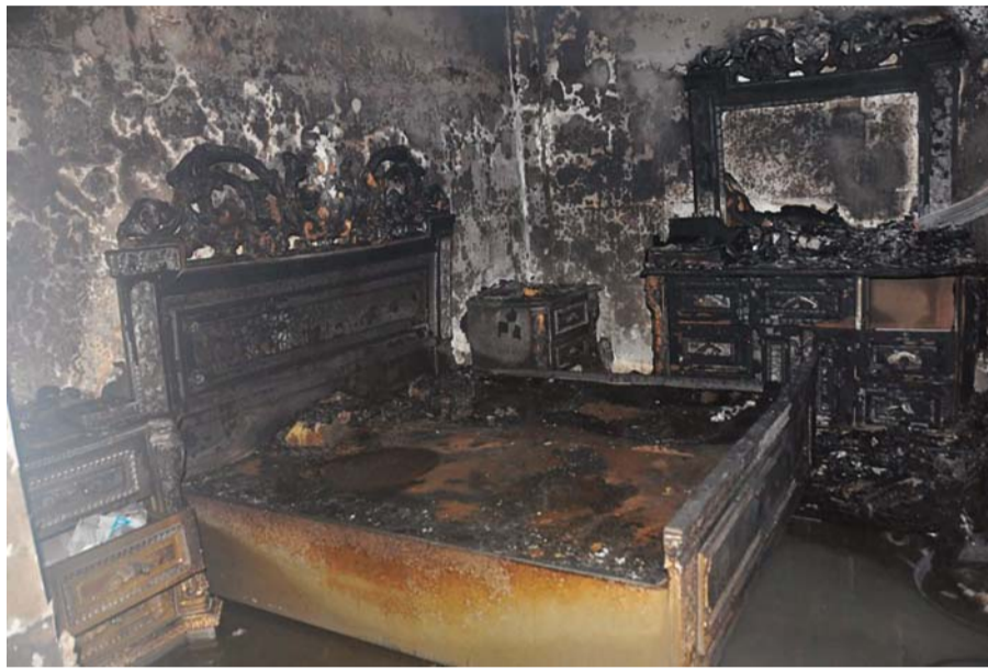
The scene inside one of the rooms in an Ardhiya house after firefighters extinguished a fire there.
