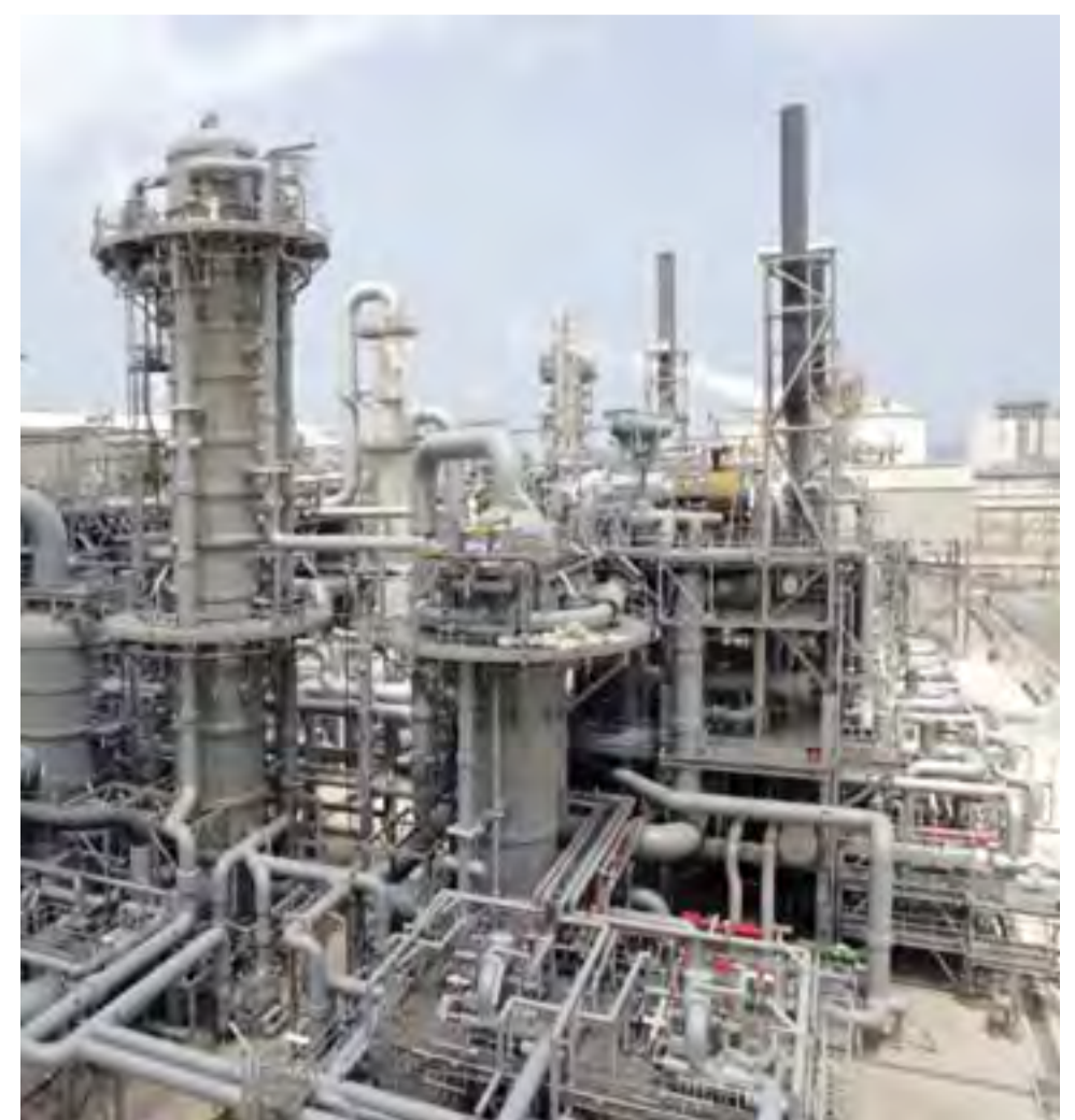
DOHA: In this April 4, 2009 file photo, a gas production facility is seen at Ras Laffan, Qatar. Natural gas exports may help Qatar protect it in the ongoing dispute it has with other Arab nations. — AP
