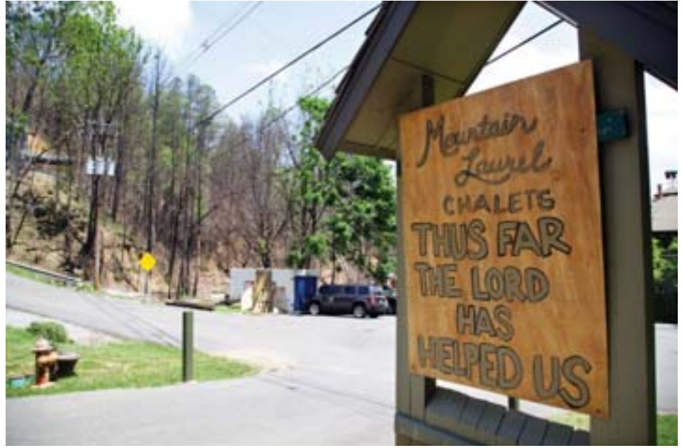
A handmade sign stands in front of the fire-damaged Mountain Laurel Chalets. — AP photos
