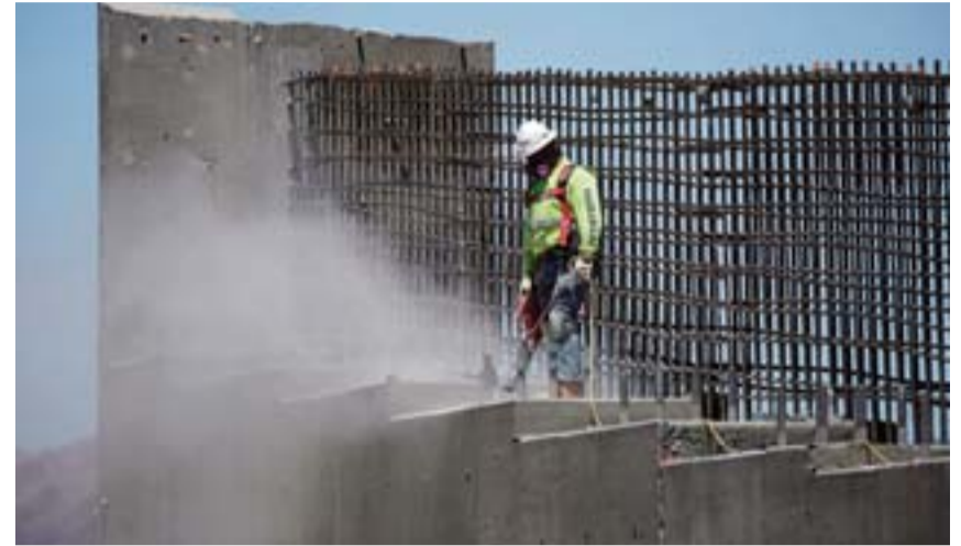
BOULDER CITY: In this May 19, 2017 photo, a man works on the Southern Nevada portion of US Interstate 11 near Boulder City, Nevada. President Donald Trump is planning a major push next week to promote a $1 trillion rebuilding of the nation's roads and bridges as his agenda has struggled in Congress and been overshadowed by White House controversies. —AP
