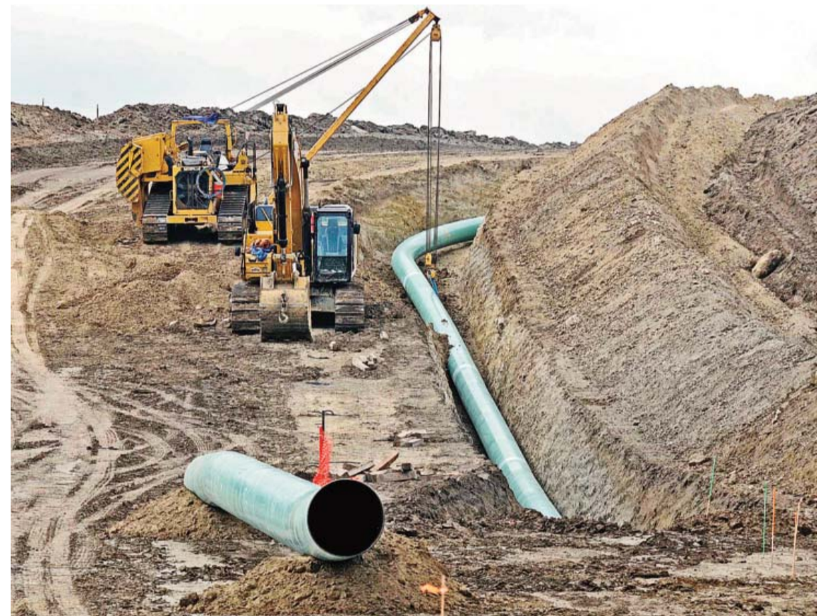
In this Oct 5 2016, file photo, heavy equipment is seen at a site where sections of the Dakota Access pipeline were being buried near the town of St Anthony in Morton County, ND. —AP
