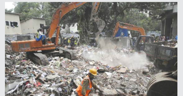
MUMBAI: Rescuers look for survivors on the second day after a five-storey building collapsed in the Ghatkopar area. —AP
