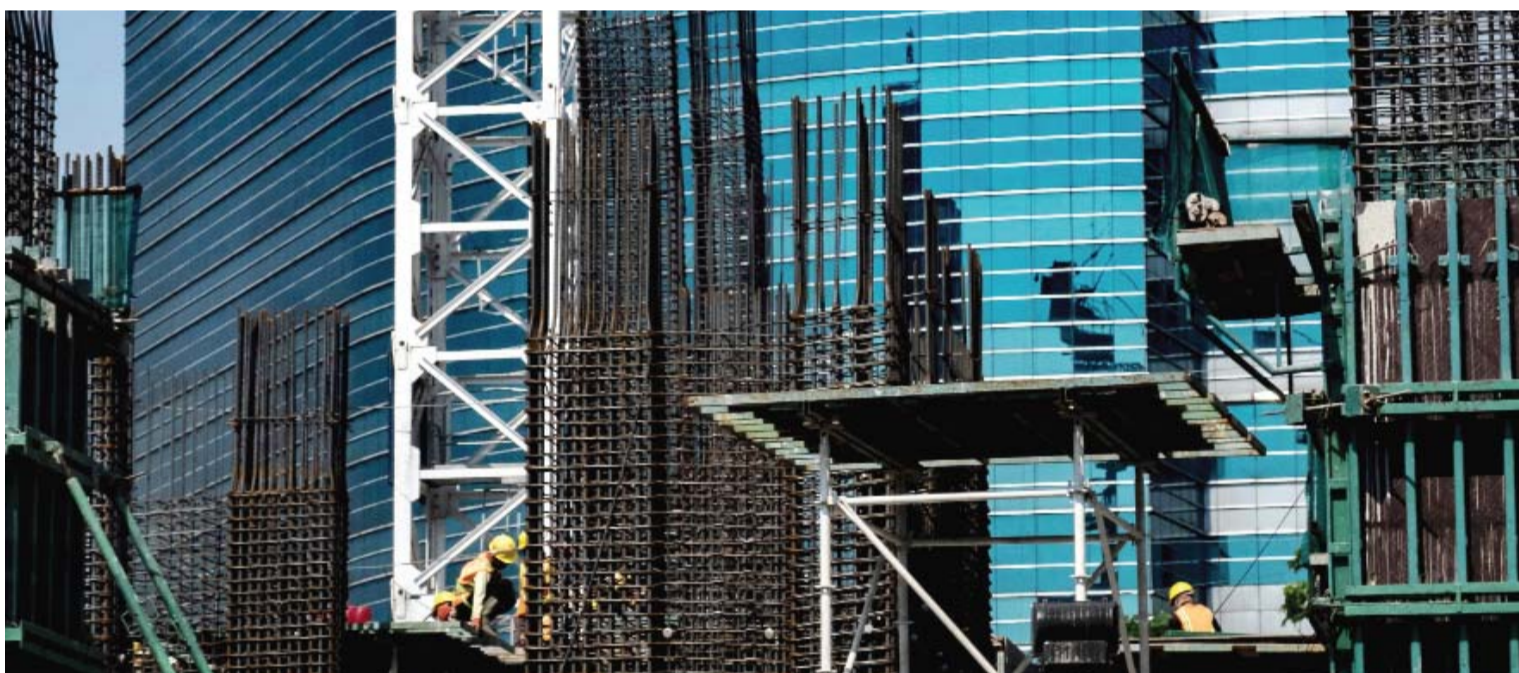
JAKARTA: Workers are seen on a building construction site in Jakarta yesterday.—AFP
