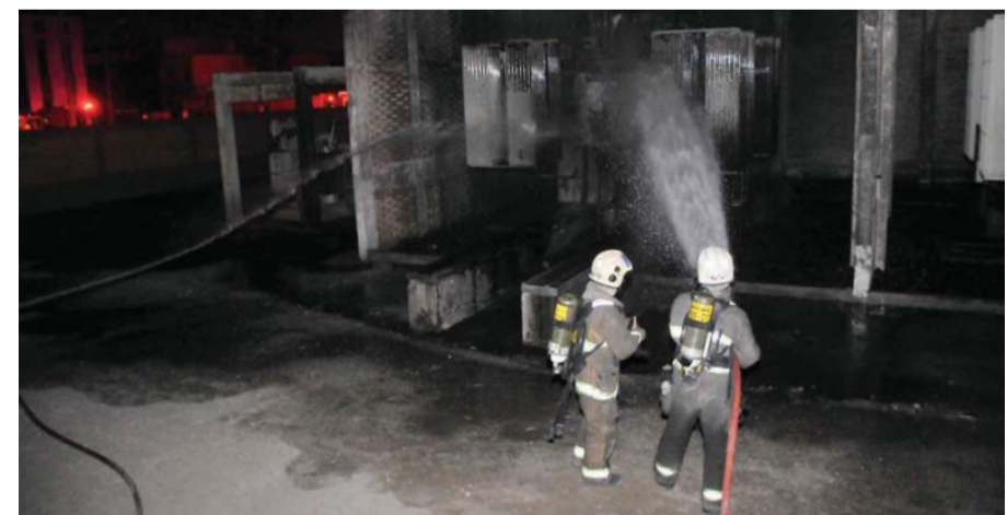
KUWAIT: Firefighters tackle a transformer's blaze.
