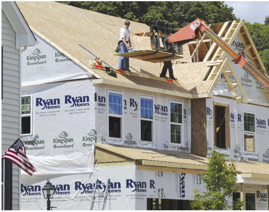
Builders work on the roof of a home under construction at a housing plan in Jackson Township, Butler County, Pa. The Commerce Department reported on US home construction in June. —AP
