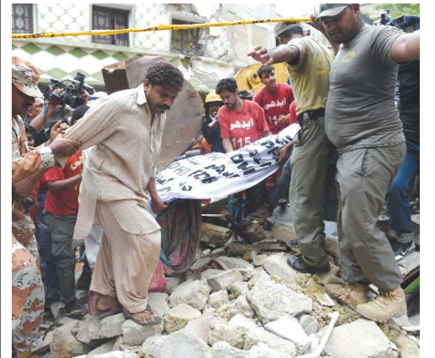
KARACHI: Pakistani rescue workers move the body of a victim from the rubble of a collapsed three storey building in a residential area. —AFP
