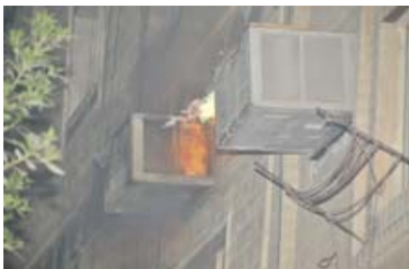
KUWAIT: Flames coming out of an air conditioner outside a Khaitan building.
