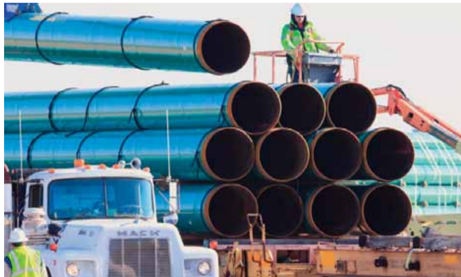
NORTH DAKOTA: In this file photo, workers unload pipes for the proposed Dakota Access oil pipeline that would stretch from the Bakken oil fields in North Dakota to Illinois. The Dakota Access project, which is mostly completed, has created about 12,000 construction jobs, according to project leader Energy Transfer Partners LP. Most of those jobs are over, however. —AP
