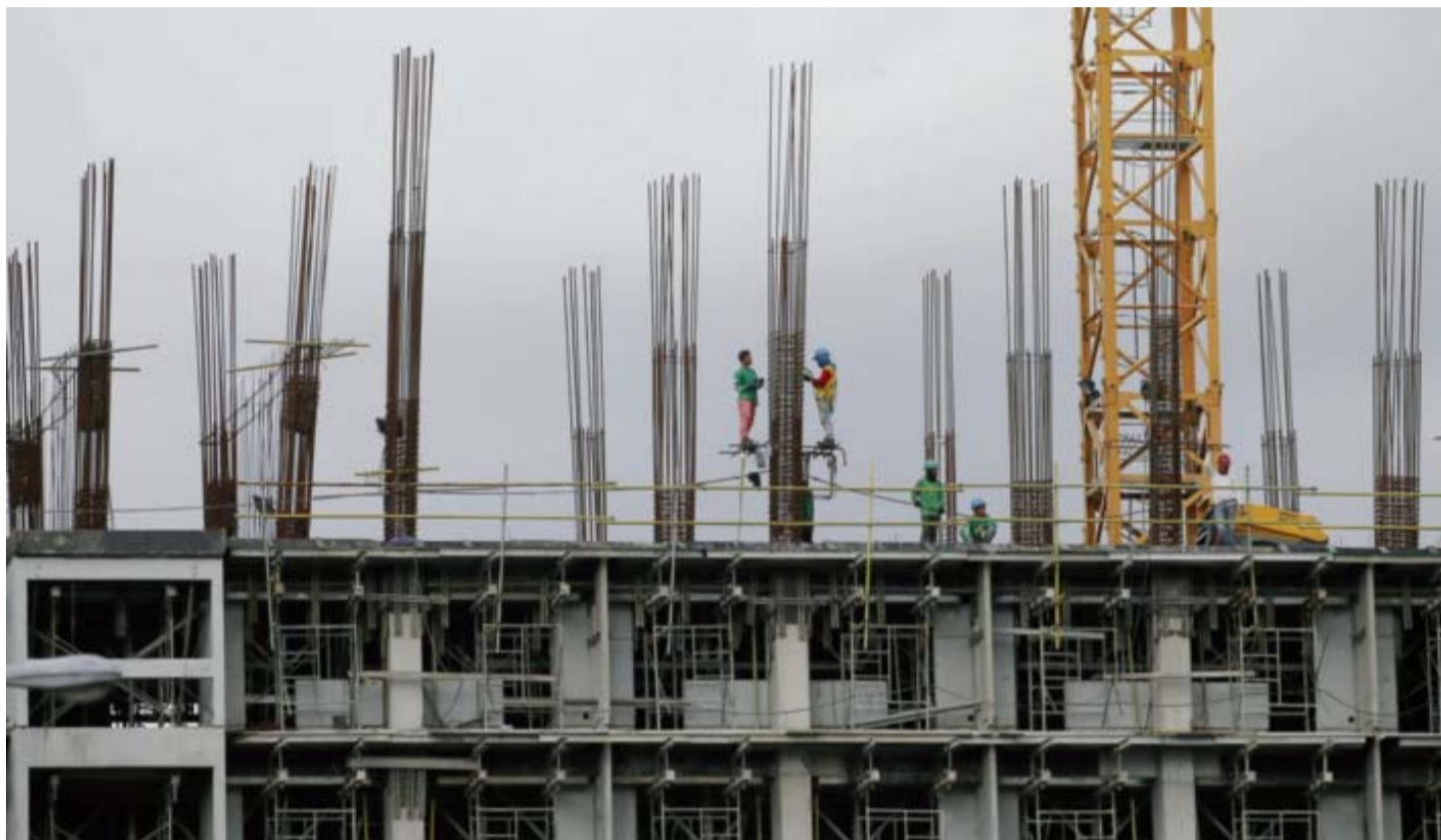
MANILA: Construction workers stand on the scaffolding around metal rods of a new pillar as they build more floors at a reclamation site in suburban Paranaque city, south of Manila, Philippines yesterday. — AP
