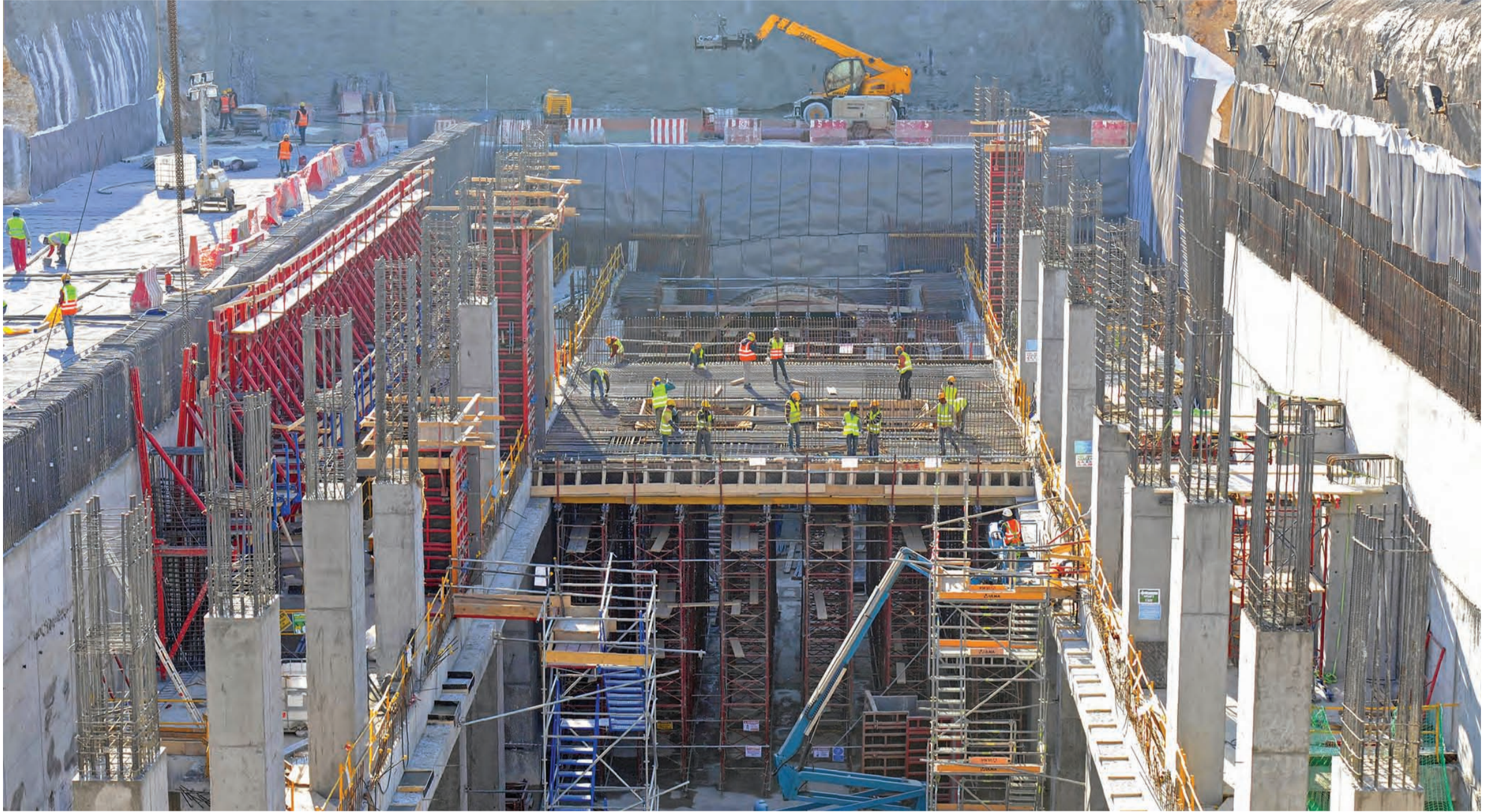
RIYADH: A general view of the construction site under the contract of French company ALSTOM as part of the Riyadh metro main line in the Saudi capital. — AFP
