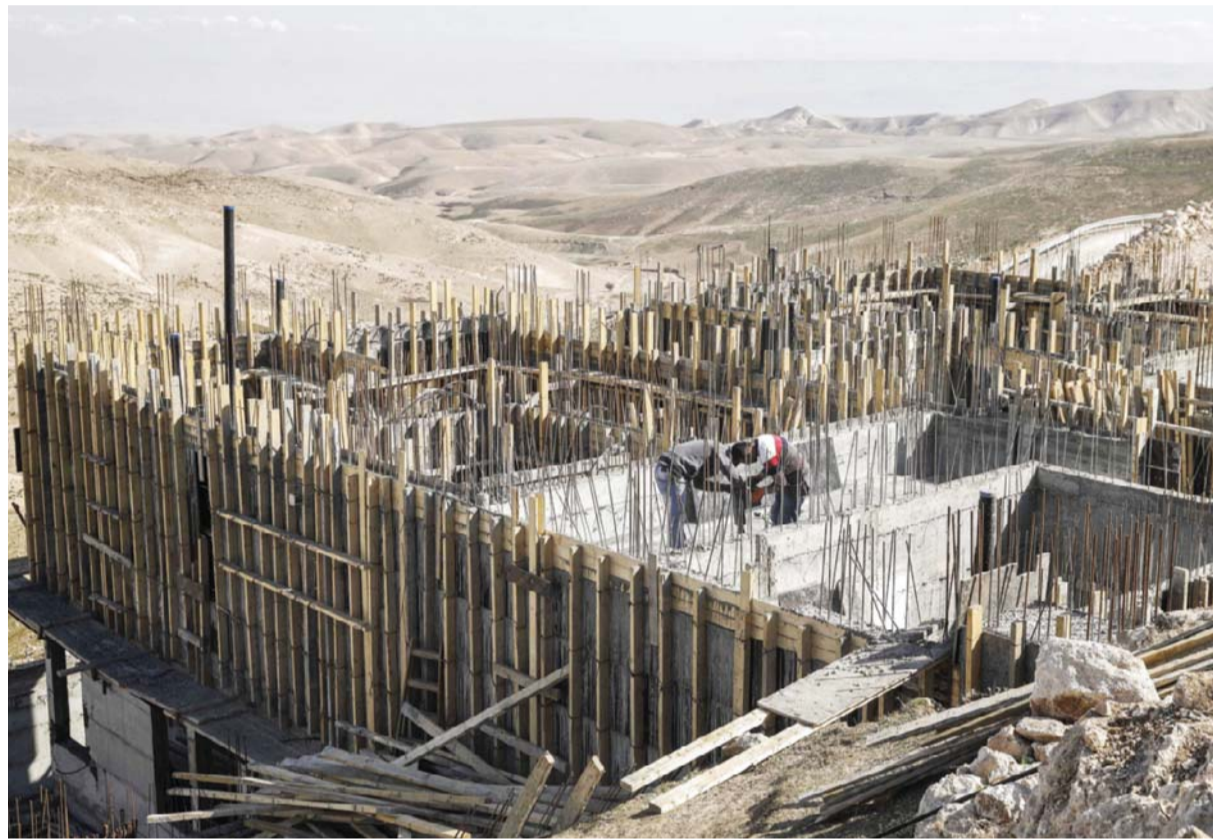
Palestinian laborers work at a construction site in a new housing project in the Israeli settlement of Maale Adumim, east of Jerusalem, yesterday. — AFP
