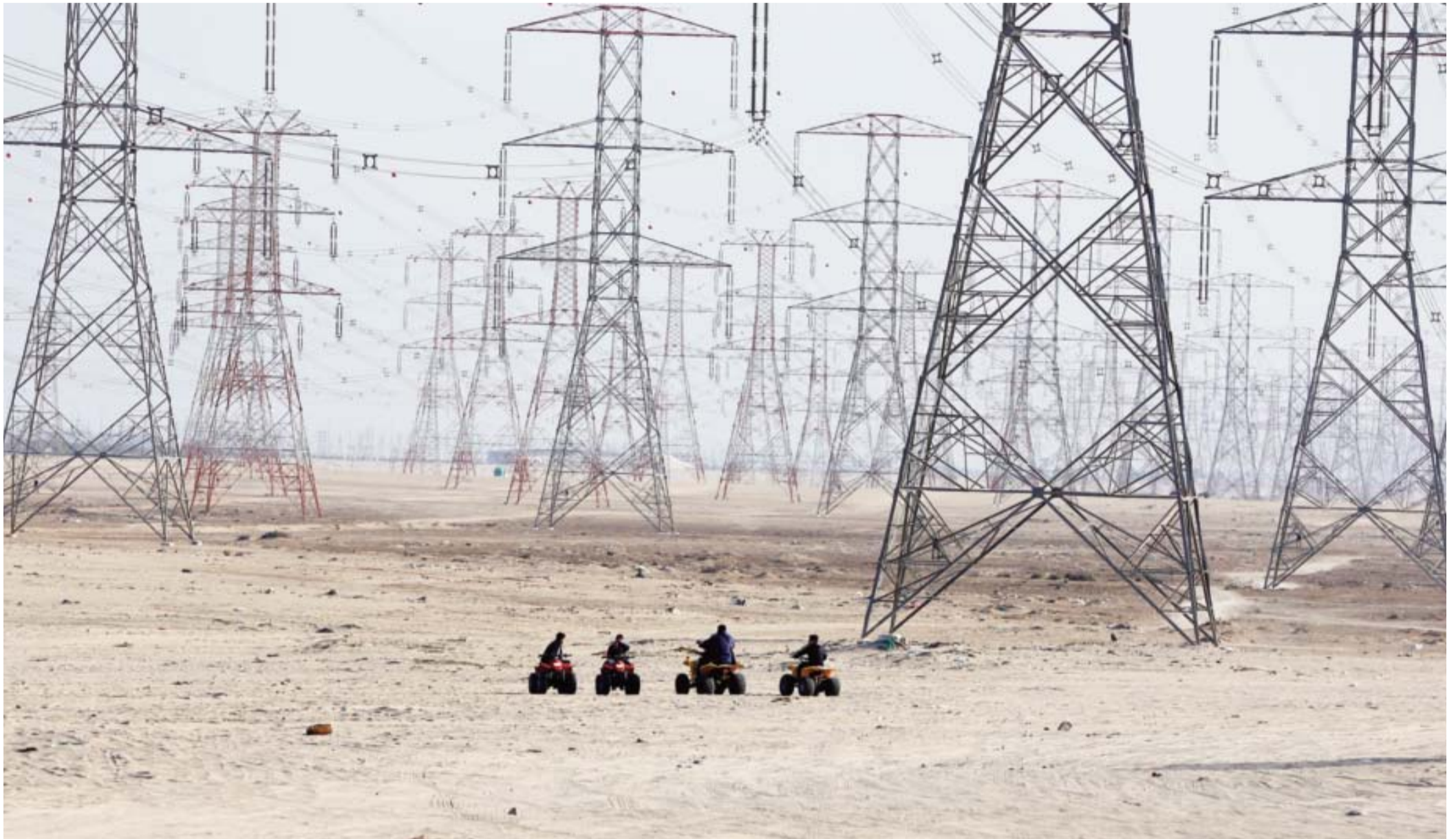
KUWAIT: Young men ride their all-terrain vehicles away from their camp and close to high voltage overhead power line transmission towers at a location north of Kuwait. Camping sites are designated in specific areas in Kuwait's desert in order to help campers stay away from military, oil and other facilities of sensitive nature. The camping season concludes on March 31, 2017.
