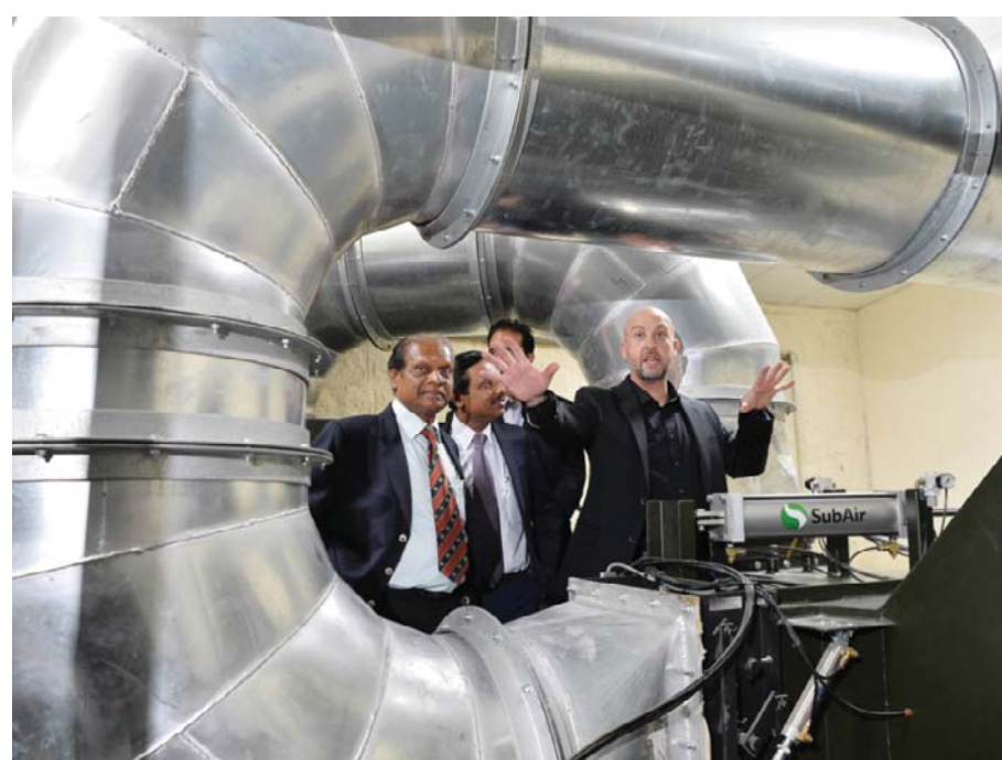
BANGALORE: KSCA officials listen as the senior vice president, Kevin Crowe (R) explains the functioning of the newly installed subsurface aeration and vacuum-powered drainage system at the Chinnaswamy Cricket Stadium in Bangalore yesterday. The system automatically kicks into action the minute it starts raining and sucks water through vacuum pipes installed underneath the outfield at a rate of 10,000 litres per minute thus avoiding match delays or cancellations. — AFP
