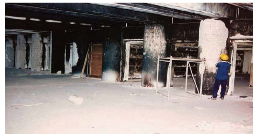
Heavy damage inside the National Assembly's building.
