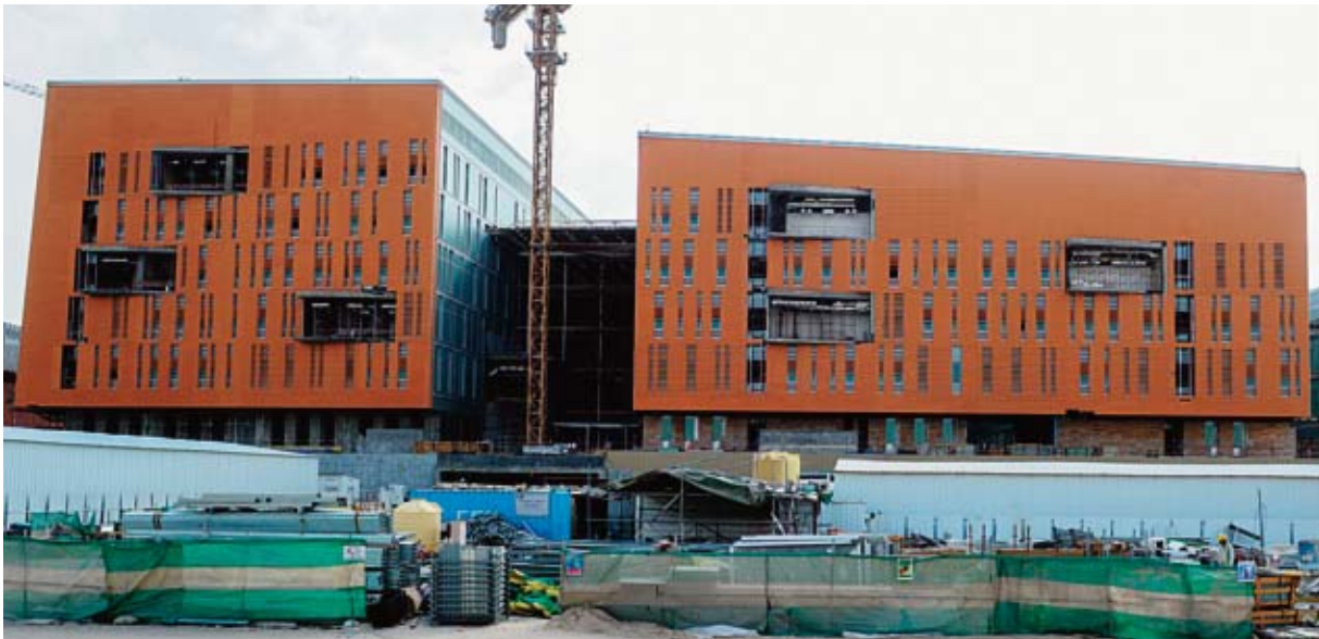
The college of engineering and petroleum at the Sabah Al-Salem University City.
