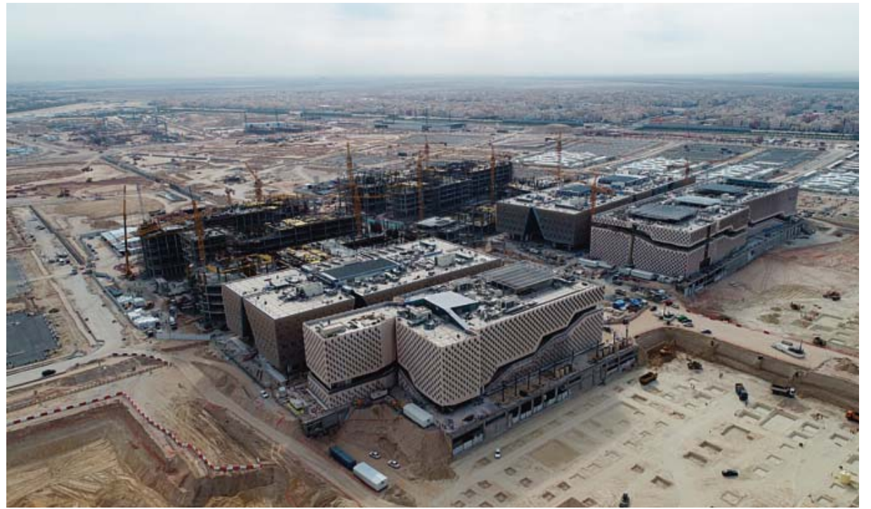
Ongoing construction works at the college of education at Sabah Al-Salem University City.
