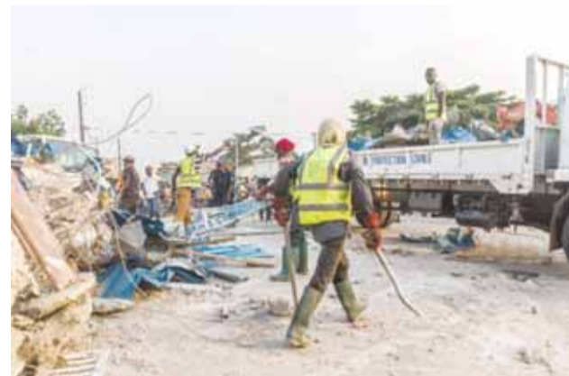
COTONOU: Workers demolish illegal structures as Benin security forces stand at a busy intersection during an evacuation in downtown Cotonou on Jan 27, 2017. — AFP
