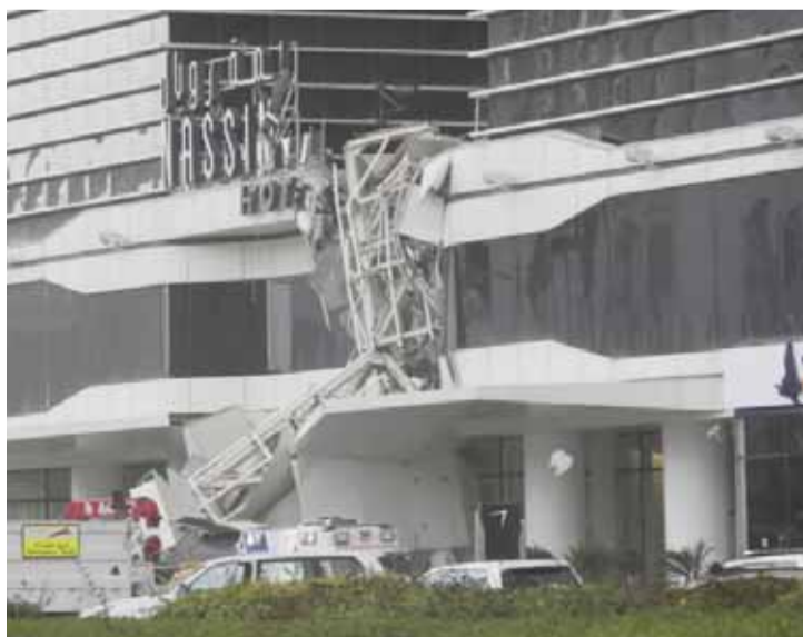
DUBAI: A construction crane is seen collapsed during high winds yesterday on the main highway running through Dubai, disrupting traffic in the heart of the commercial hub. — AP
