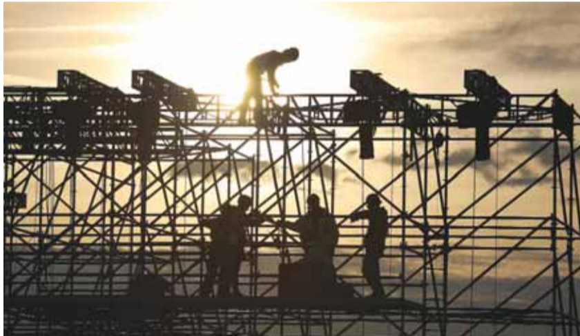
WASHINGTON: This photo taken on Jan 12, 2017 shows workers as they prepare the stage in front of the Lincoln Memorial. The US economy continued to pump out new jobs in January, adding 227,000 positions, while the unemployment rate rose a tenth to 4.8 percent. — AFP
