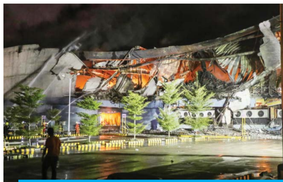
DAVAO: Firefighters extinguish a fire at a shopping mall on Saturday. — AFP
