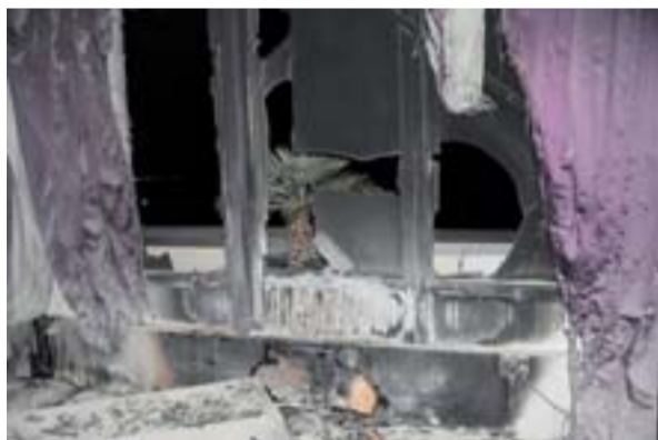
KUWAIT: Damage left by a blaze reported in a Salmiya hotel on Monday night.
