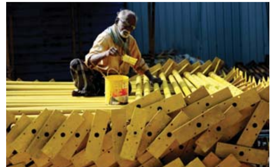
CHENNAI: An Indian laborer paints iron rods at an under-construction site yesterday. — AFP
