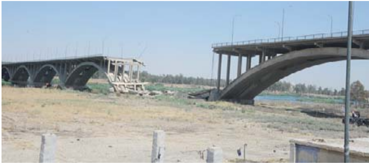
A destroyed bridge in Mosul.
