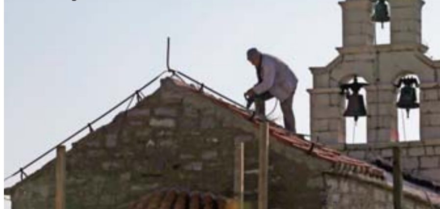
A worker repairs roof on Holy Sunday church in the 'Tsar's Village' complex near Sveti Stefan peninsula in Montenegro.
