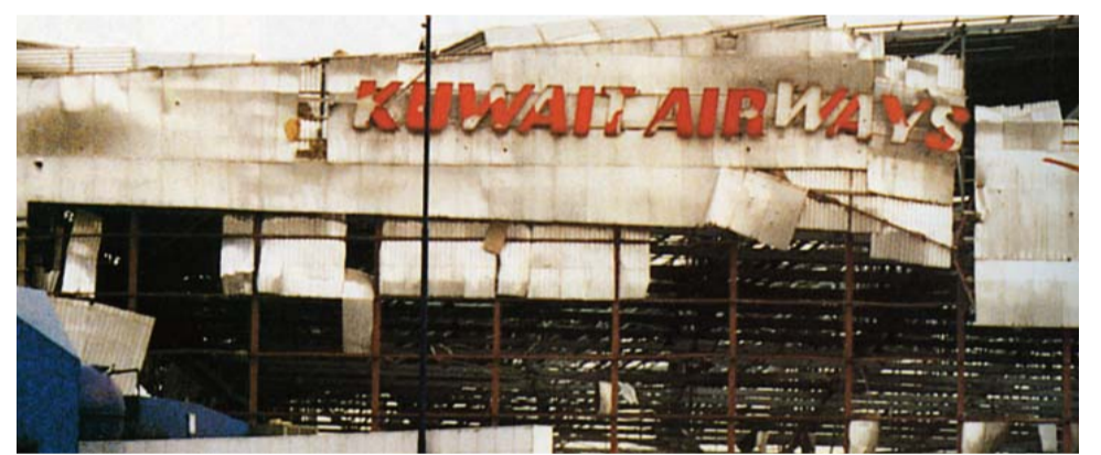
Heavy damage at Kuwait International Airport.
