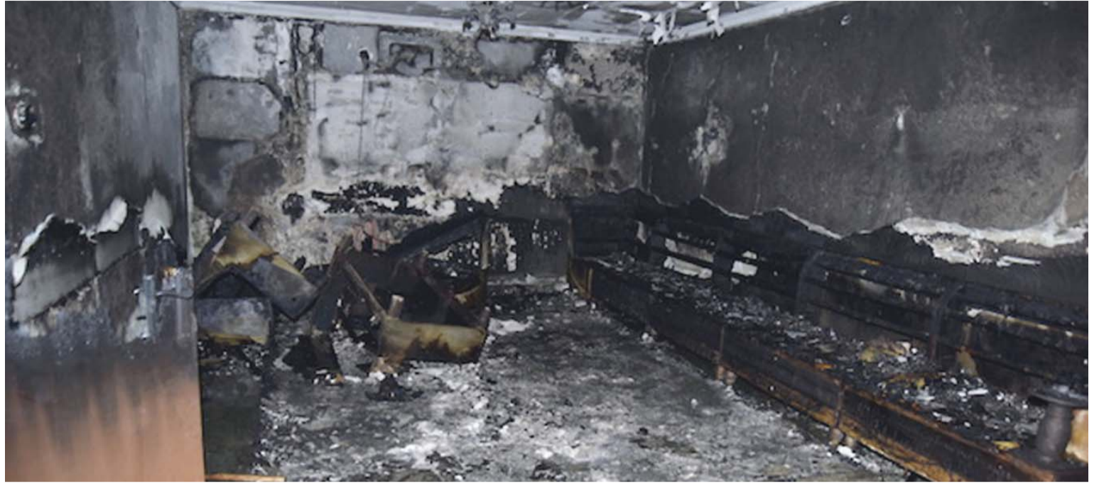
KUWAIT: Damage left by a fire reported yesterday in a Rabiya house.
