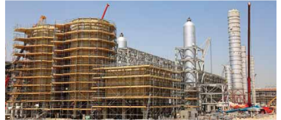
Ongoing construction works at Kuwait Petroleum Corporation's clean fuel and integrated refining complex projects.
