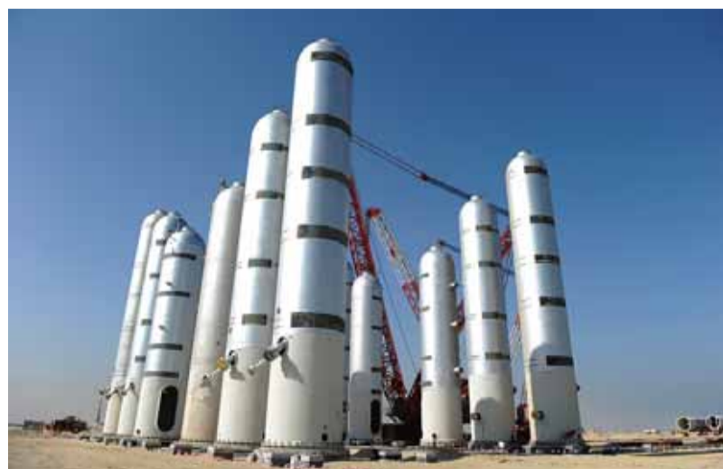
Ongoing construction works at Kuwait Petroleum Corporation's clean fuel and integrated refining complex projects.
